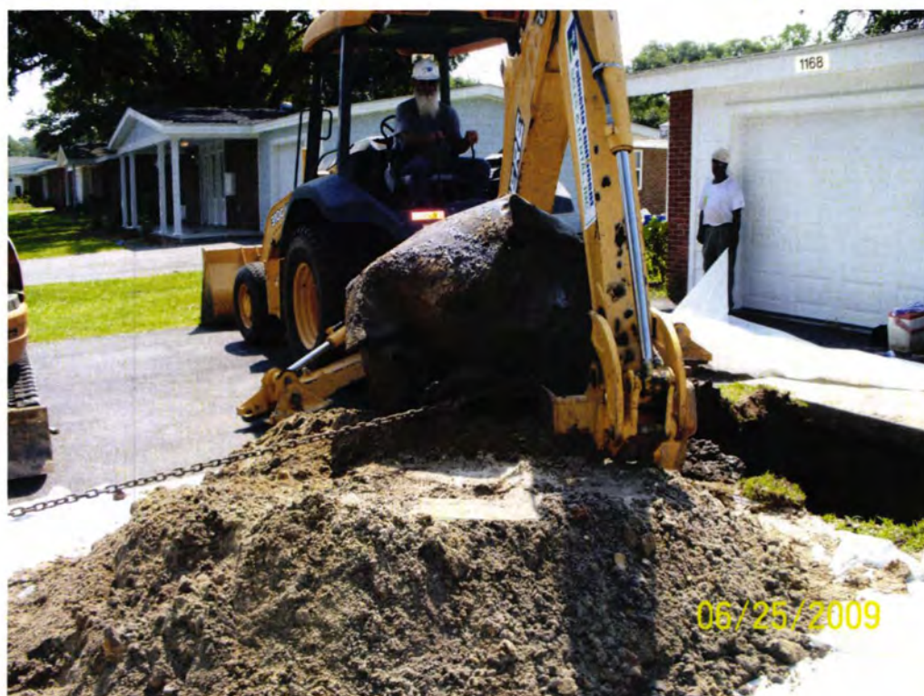
Picture 2: Crushed UST 1168Jasmine sits atop the pile of sand.
